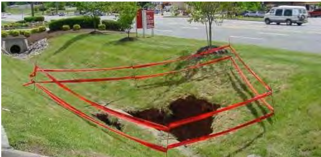
Figure 3.32. Sinkhole Collapse Adjacent to Chapman Highway, May 2005
